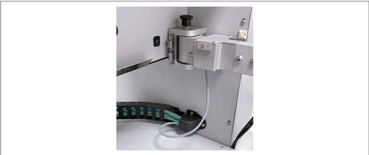
Fig. 15: Cable routing outside the housing, picture after assembly completion.
