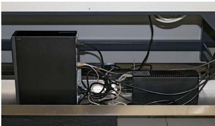
Fig. 9: PC and UPS installed
