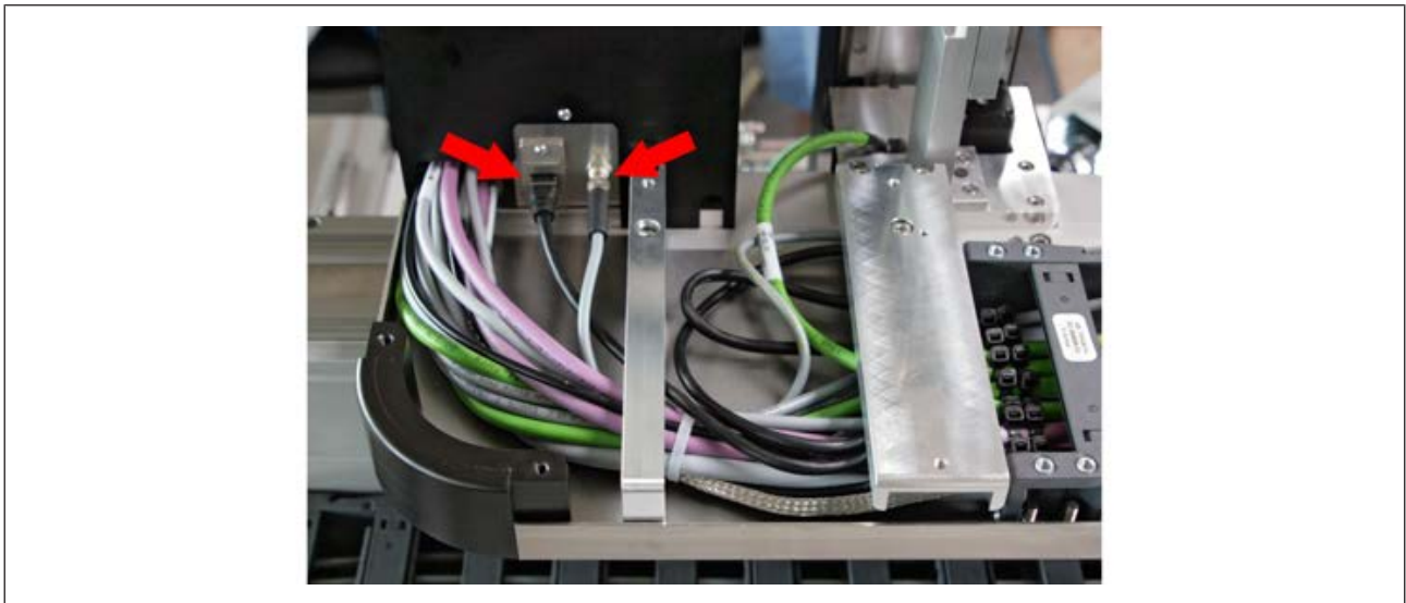
Fig. 24: Lower picture: Plug connected. Arrow on the left: Ethernet cable, arrow on the right: Lighting
